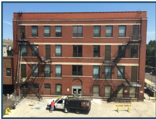
This summer a crew repaired and painted the emergency stairs on the outside of our school’s east building.
