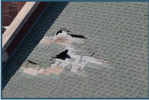
Winds ripped shingles off the church roof in several locations last September. A generous donor helped us to make repairs immediately.
